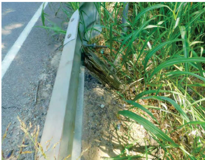
SPAN 4 RIGHT GUARD RAIL POST HAS HEAVY DECAY
