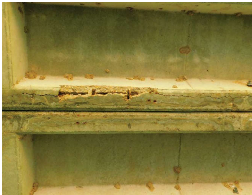
SPAN 3 PCCS B SPALLING TO STEEL
