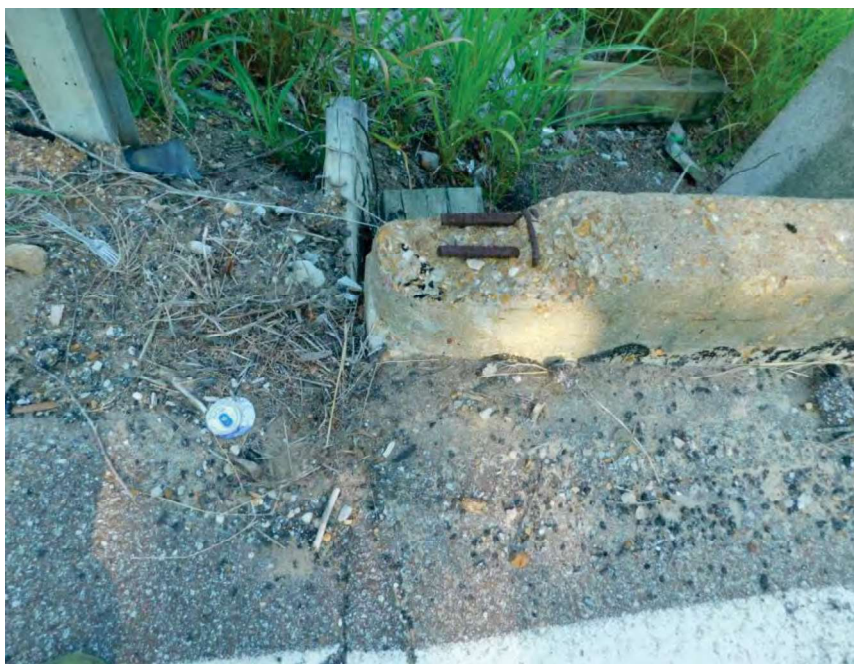
SPAN 1 CURB SPALLING TO STEEL (LEFT CURB)
